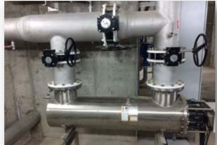
UV reactor (16 lamps)
