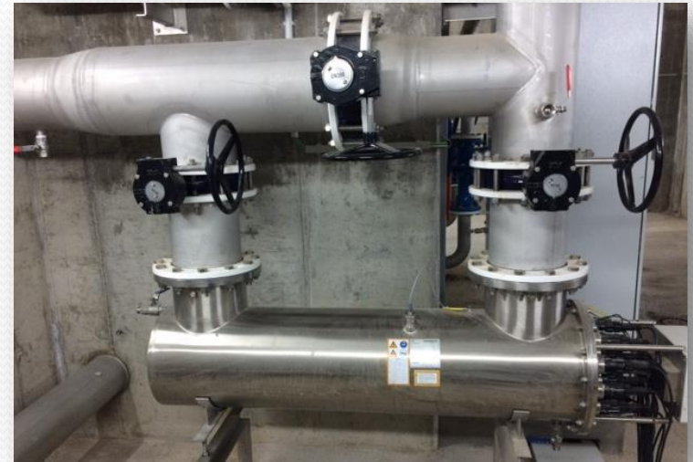
UV reactor (16 lamps)
